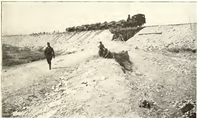
A PORTION OF THE NEVERS CUT-OFF — A PIECE OF RAILWAY CONSTRUCTION IN FRANCE UPON WHICH A NUMBER OF TECH MEN WERE ENGAGED
